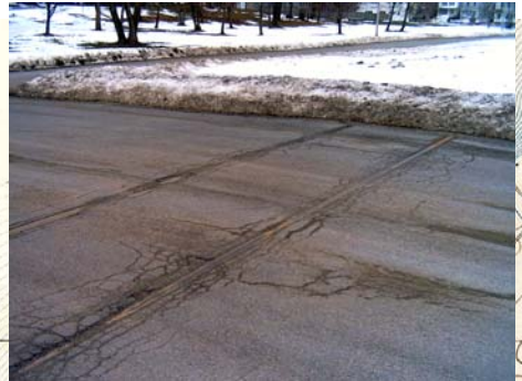
O&W RAILS in Pavement
